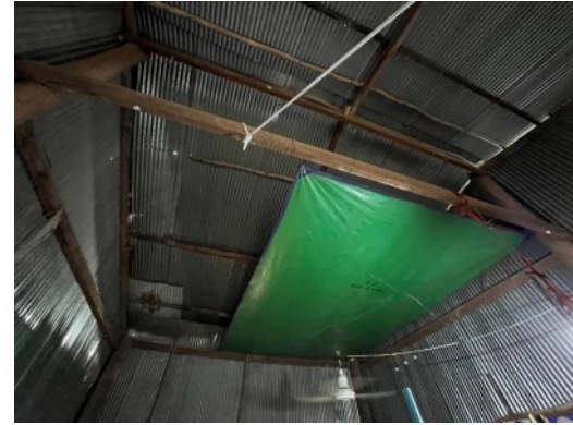
Sreymao is using the green tent to keep her house dry from leaking roofs.
